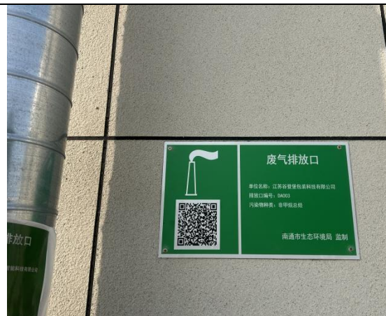
DA003/18m 排气筒标志牌
