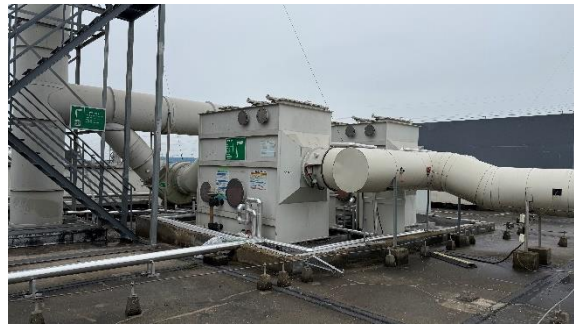
DA003 标志牌及配套一级碱喷淋塔
